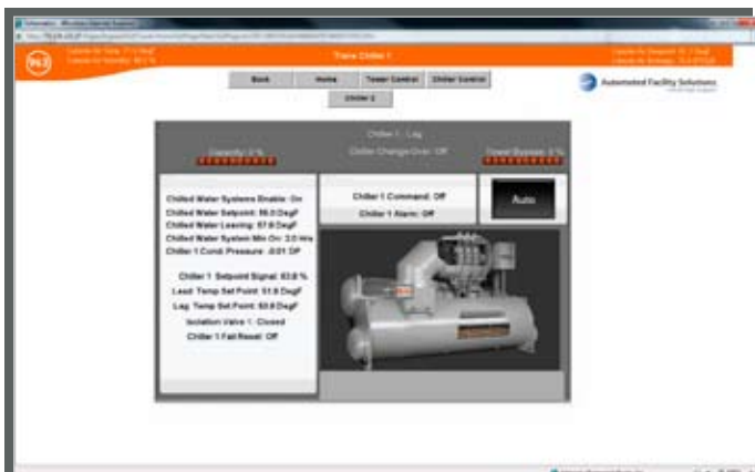
A Trane chiller integrated into the Quintiles building controls system: The Trend system delivers accurate, real-time building data for precision control of the facility.
