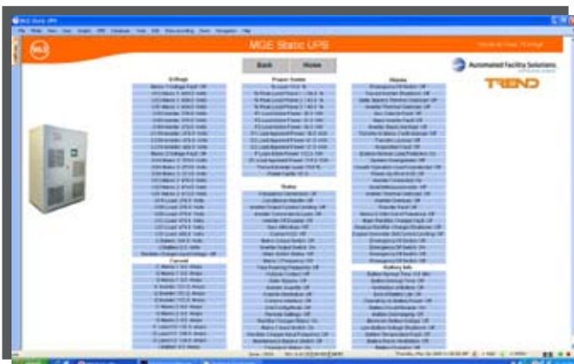
One of the status uninterruptible power supply (UPS) units; Trend's 963 Supervisor front end centralizes control of all the different building systems and devices.
